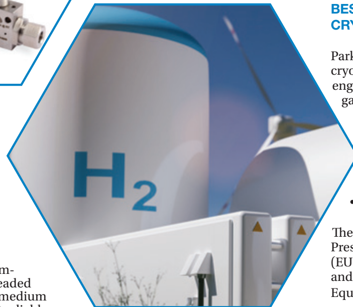
Hydrogen storage tanks, compressors and pressure control devices
